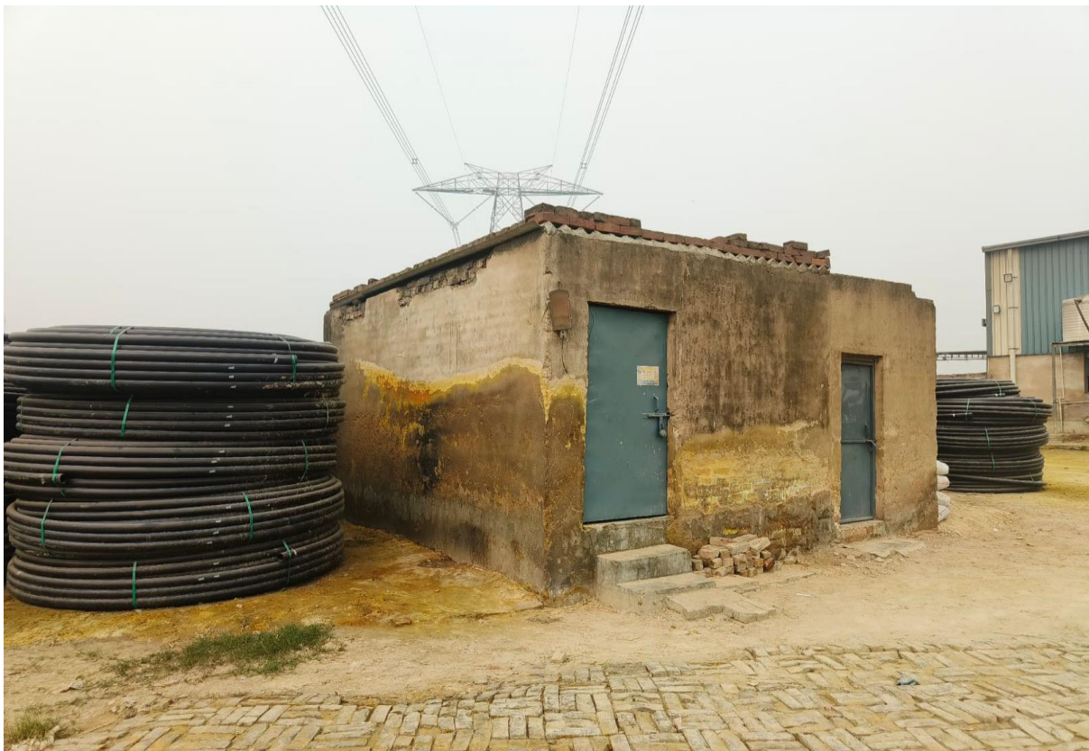
Image 28: Impact of chromium in soil & groundwater on the buildings
