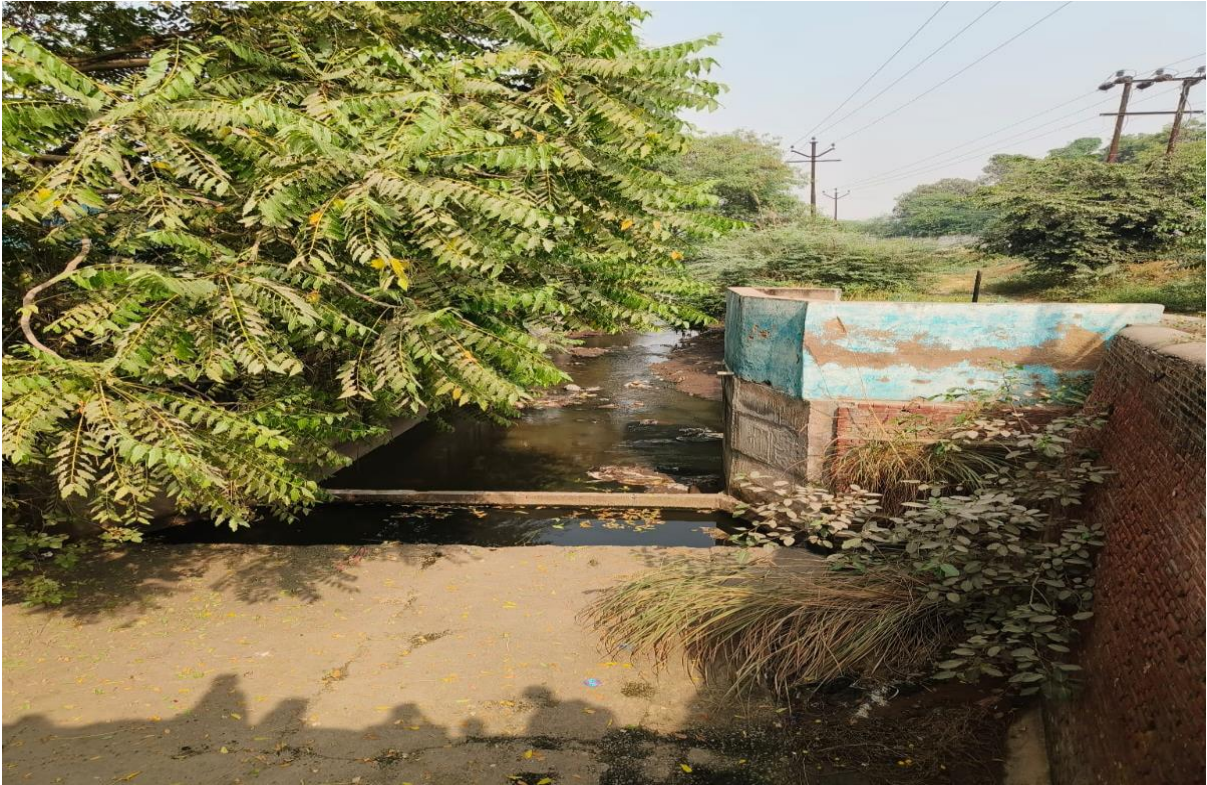
Image 10: pumping point of the COD drain (into Bingawa STP)
