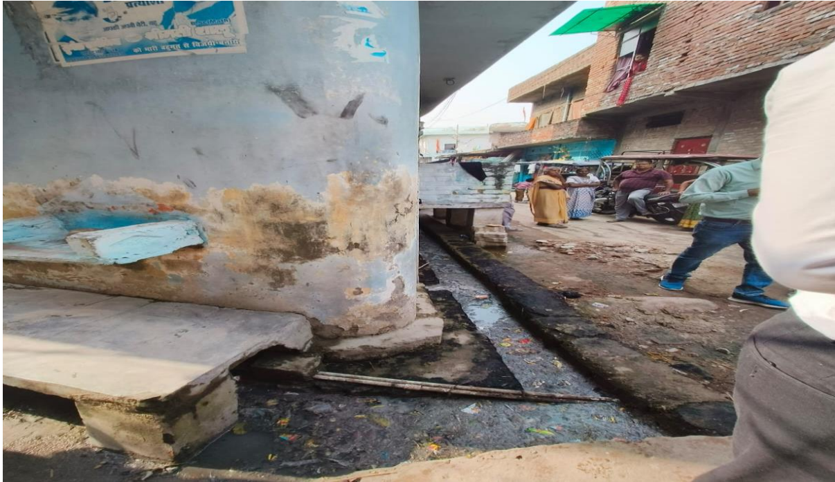
Image 12: Juhi baburiya choked sewage lines
