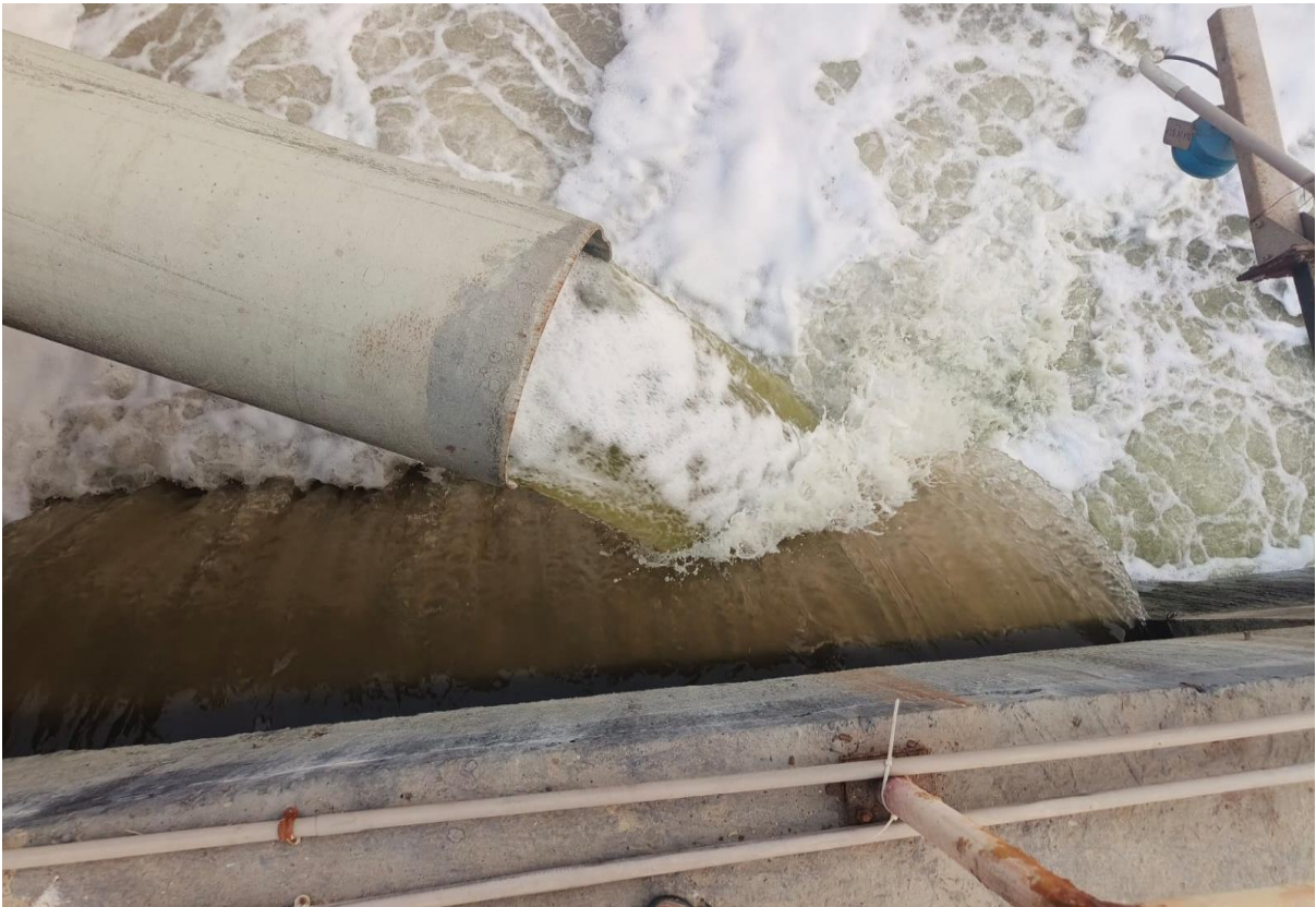
Image 17- Outlet of 36 MLD STP (previously CETP)
