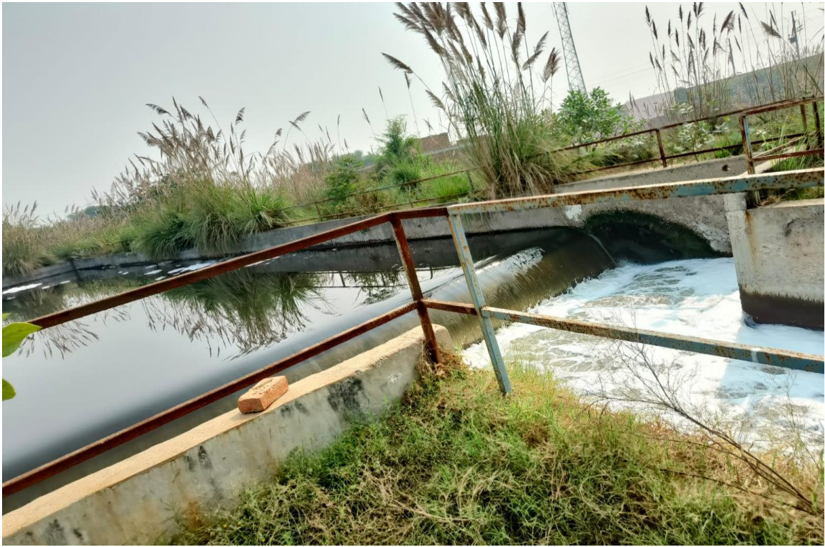
Image 6: outlet point of the STP (After chlorination)
